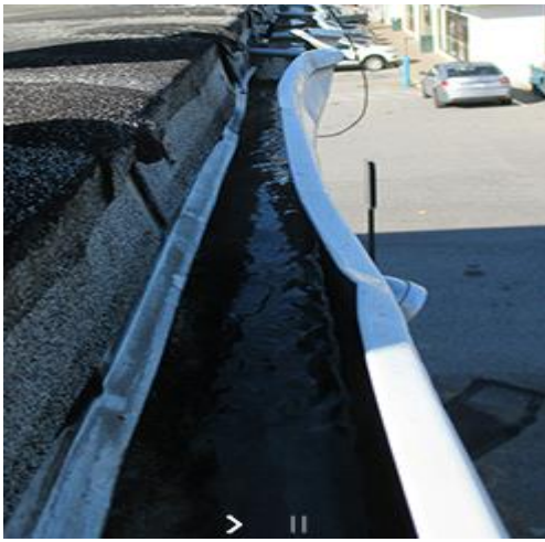
THIS RESIDENTIAL GRADE GUTTER ON A COMMERCIAL BUILDING HAS BEEN BENT AND DAMAGED.
