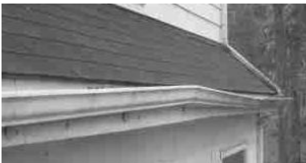
IMPROPER SLOPED GUTTER.
