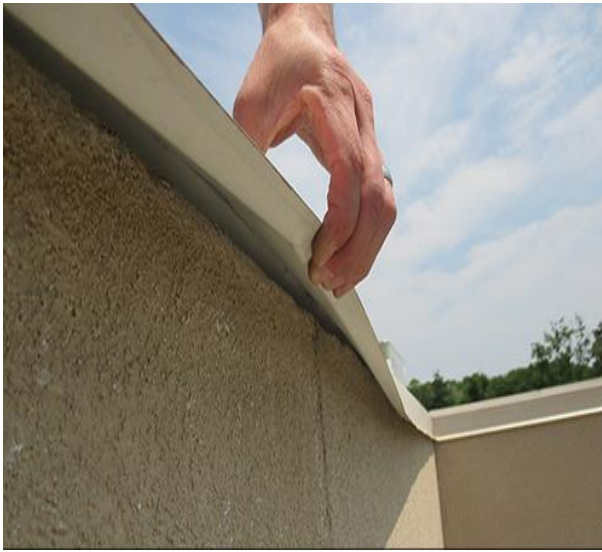
LIGHT GAUGE OR RESIDENTIAL METAL EDGING CAN EASILY BEND. THIS APPLICATION IS ALSO MISSING CONTINUOUS CLEATING.
