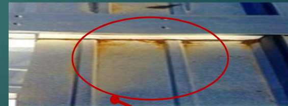
Failure to Remove Cutting Debris (Swarf) Quickly Causes Panel Corrosion, Staining and Rust.
